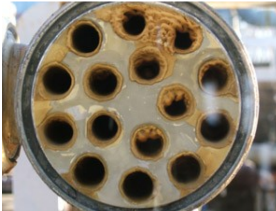
Abattoir Heat Exchanger: Before installing a Conditioner
