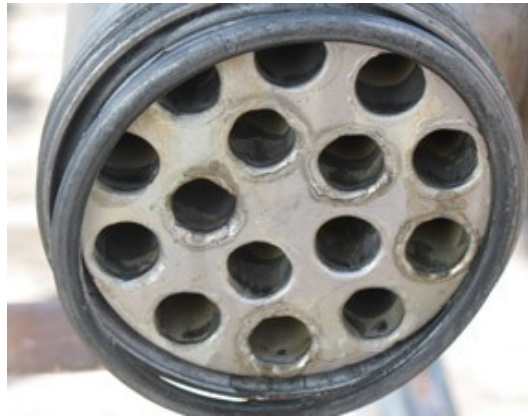
Abattoir Heat Exchanger: AFTER installing a Conditioner
