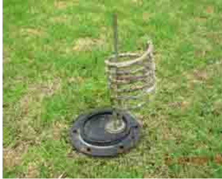
Hot Water Element: AFTER installing a Conditioner
